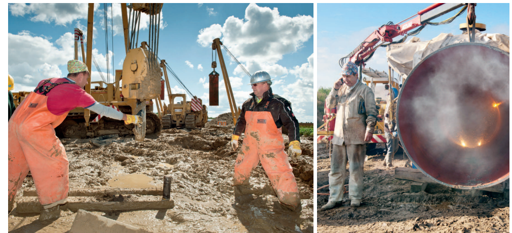
PIPING UP: New natural gas pipelines are laid near Pilsen, Czech Republic (top) and in Mecklenburg-Vorpommern, Germany (below left and right). But even such major infrastructure, delivering gas from Siberia via the Nord Stream pipeline under the Baltic, provides no guarantees in an era of new price volatility.
